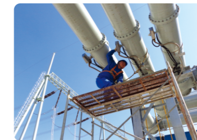
The service site of the 800kV Pu'er Converter Station of China Southern Power Grid EHV Transmission Company
