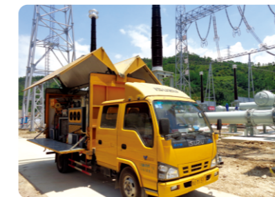
The Service Site of the 1000kV UHV Zhenan Substation of State Grid
