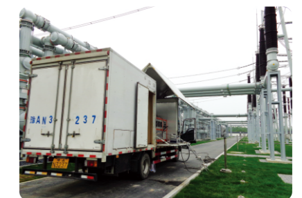
The service site of the 500kV Tongxiang Substation in Zhejiang Province
