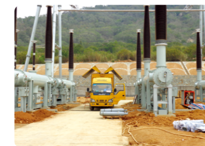
The service site of the 500kV Donggang Substation in Xiamen
