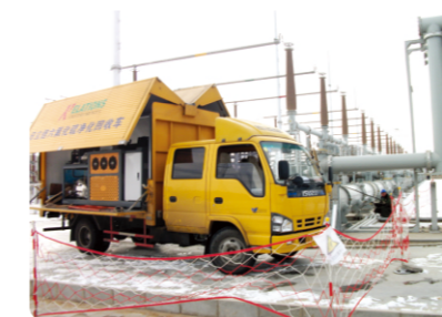
The service site of the Chaidamu Converter Station
