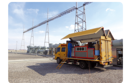
The service site of the 750kV Huanghe Substation of Ningxia Electric Power Company
